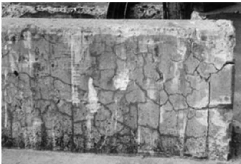
Figure 5-72 Cracks caused by AAR
